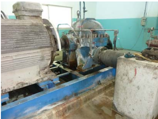
WADI-ARAB New Pumping Station No. 1
