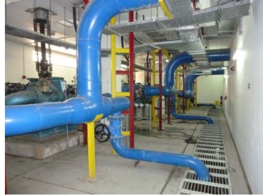
Main Pumping Station in Amman
