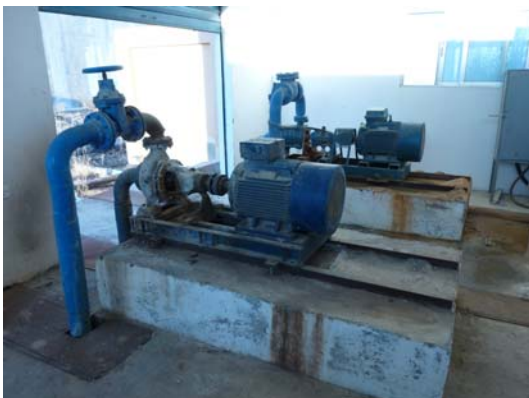
Ma'an Main Pumping Station
