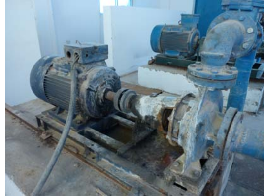
Ma'an Main Pumping Station
