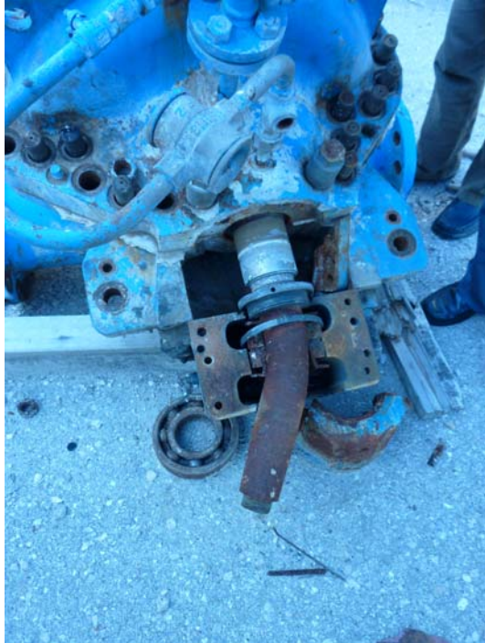
WADI-ARAB Pumping Station - Bended Shaft
