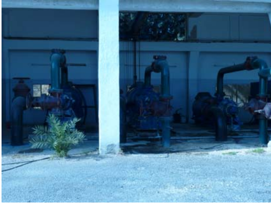
ZABDA Pumping Station
