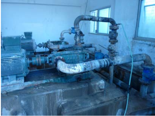
RAWAZ Booster Station
