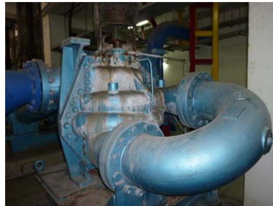
Main Pumping Station in Amman
