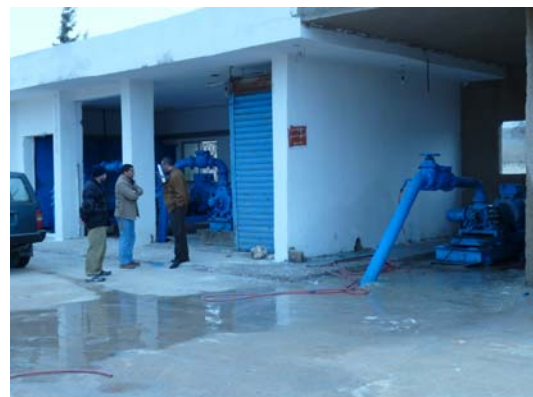
ZEBDA Pumping Station
