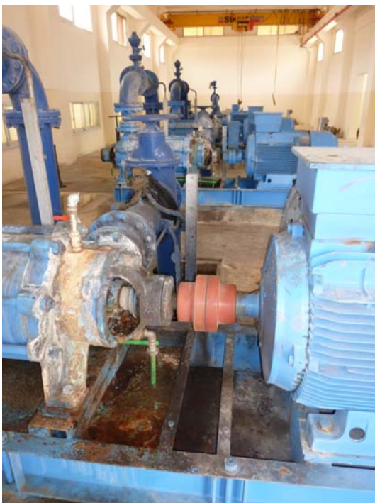
HISA Pumping Station No. 1
