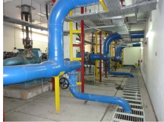
Main Pumping Station in Amman
