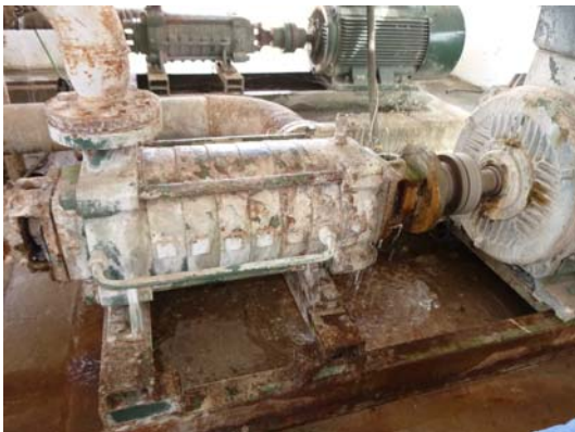
RAWAZ Booster Station
