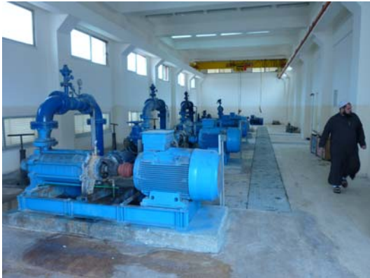
HISA Pumping Station No. 1
