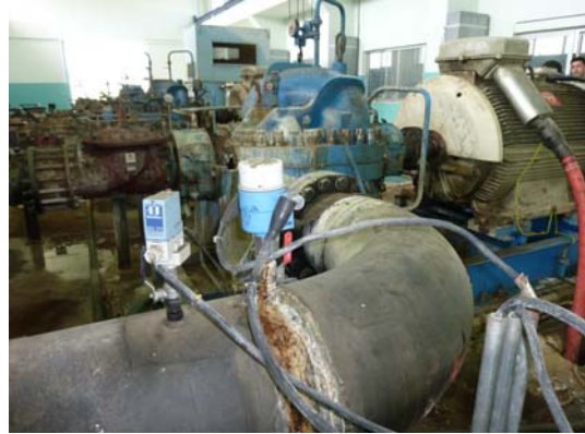
WADI-ARAB New Pumping Station No. 1
