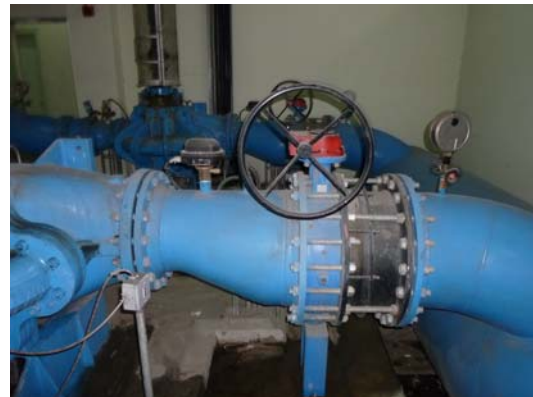
Main Pumping Station in Amman
