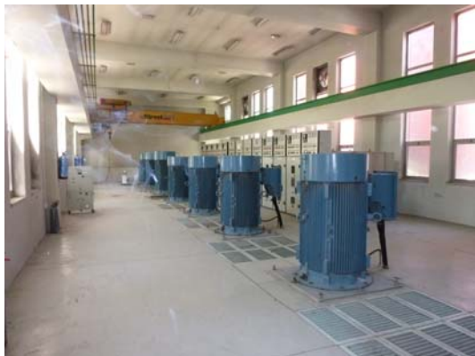
Main Pumping Station in Amman
