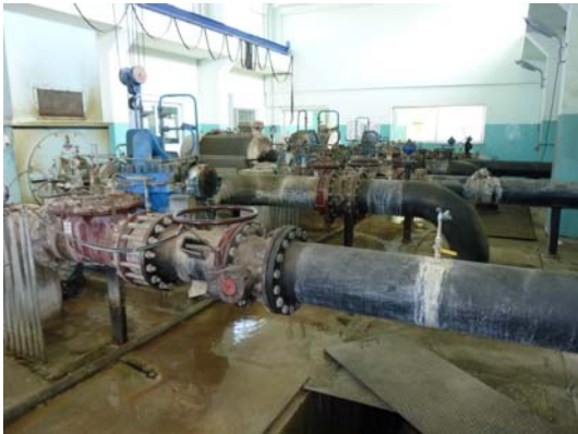
WADI-ARAB New Pumping Station No. 1
