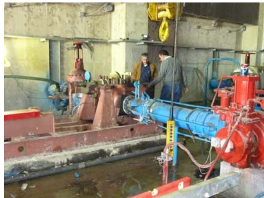
WADI-ARAB Pumping Station No. 1
