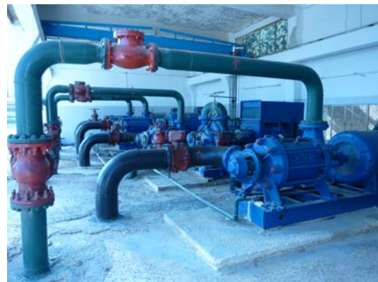
ZABDA Pumping Station
