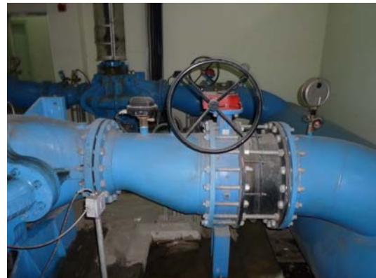
Main Pumping Station in Amman
