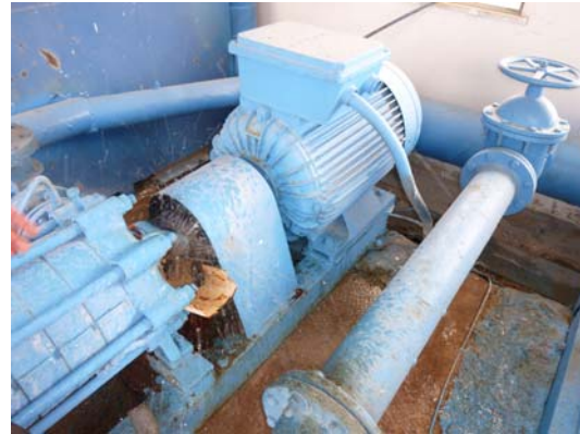
ZEBDA Pumping Station
