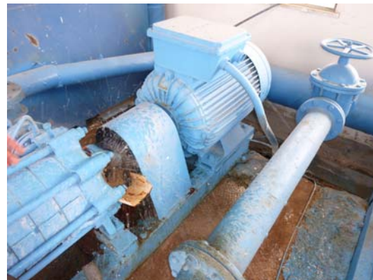
ZEBDA Pumping Station
