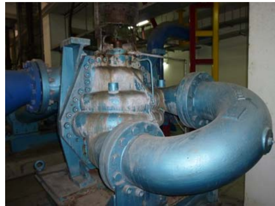
Main Pumping Station in Amman
